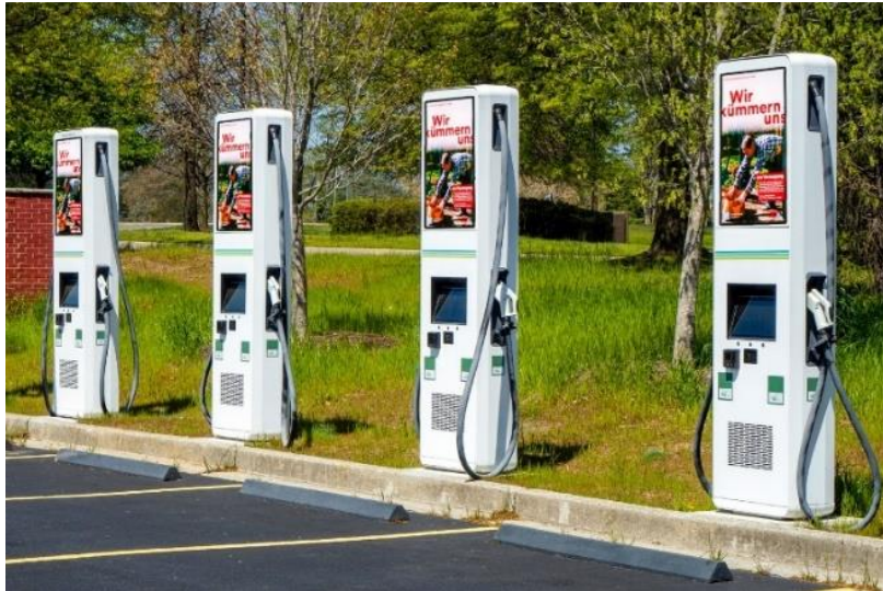
Figure 2.34: Public charging station
