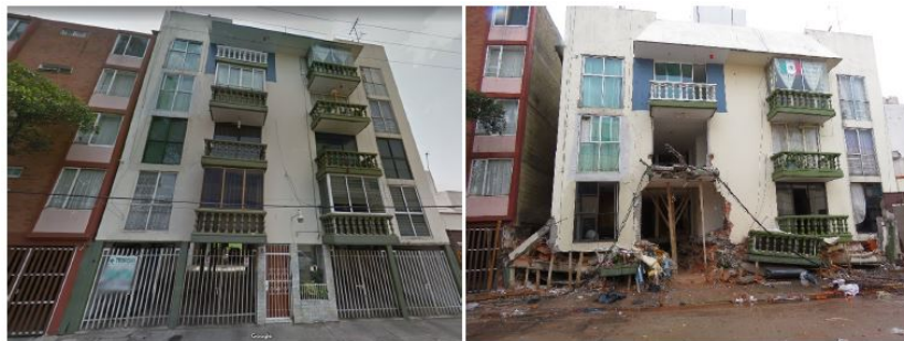
Figure 2.43: a) Residential building collapsed due to soft first story at Balsas 18, Miravalle, before the 2017 Puebla-Morelos earthquake (left) and after the earthquake (right). [From Galvis et al. (2017)].
