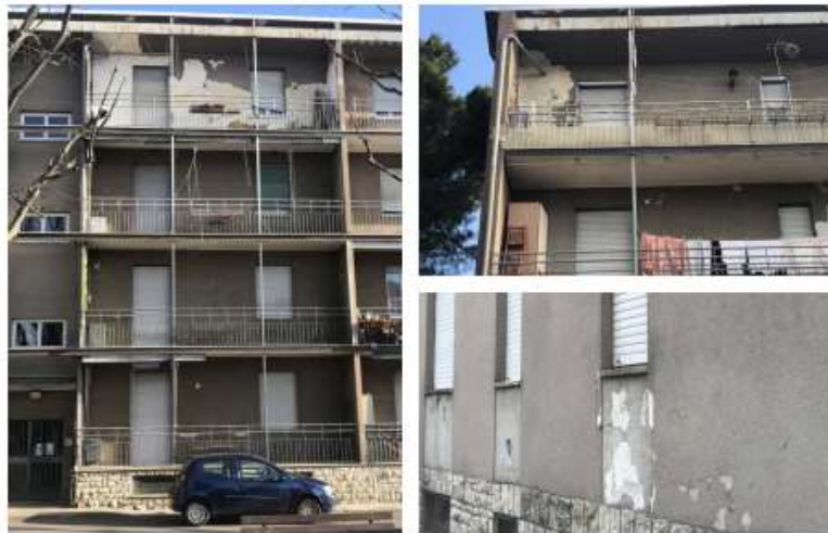
Figure 5.1: Detail of the severe degradation of the building
