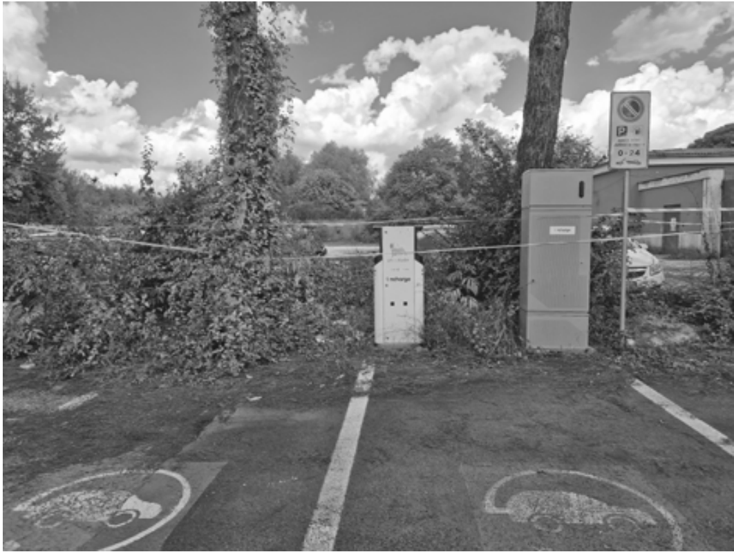
Fig. 165 A disused charging station
