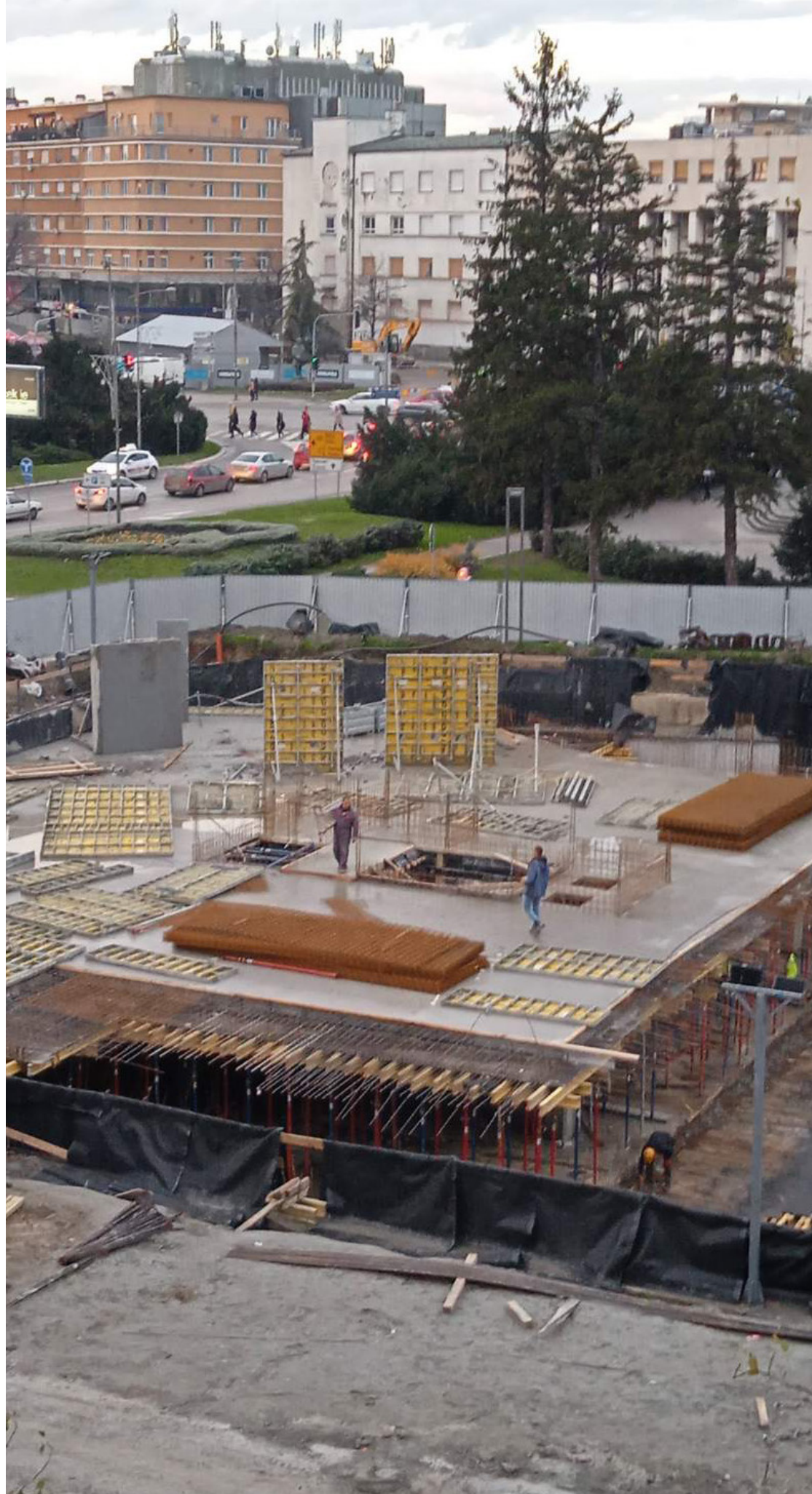
Figure 3.10 (left) Works on the construction of a parking lot in the city center (Source: gradnja.rs)
