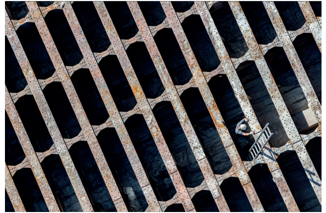
Figure 18. View of where the High Line's original concrete deck was removed, revealing the historic steel beams below.
