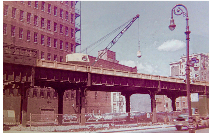
Figure 5. High Line Demolition- crane with wrecking ball mounted on the trestle. Photo by Peter H. Fritsch (1962).
