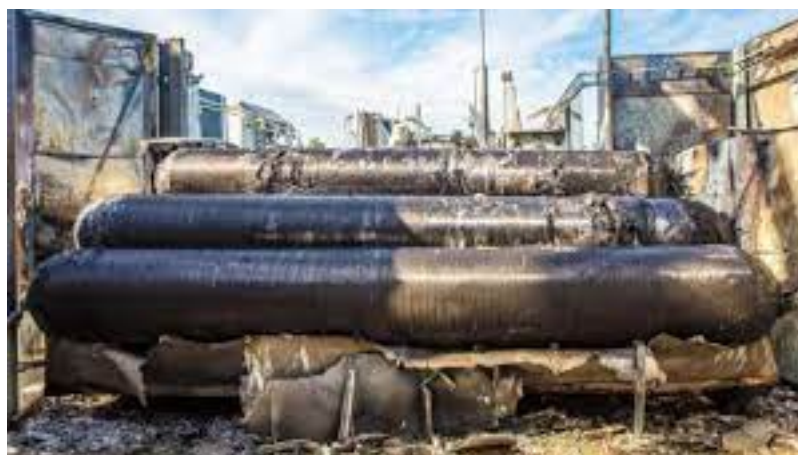
Figure 3.4: Tanks of the refueling station of Kjørbo
