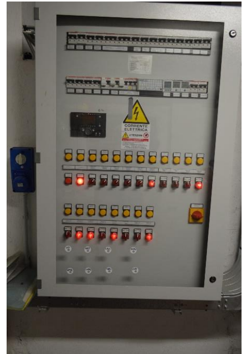
Figure 90: the electric panel
