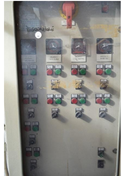
Figure 105 The electric panel
