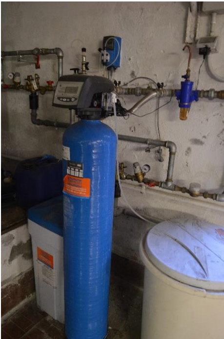
Figure 89: the water softener system
