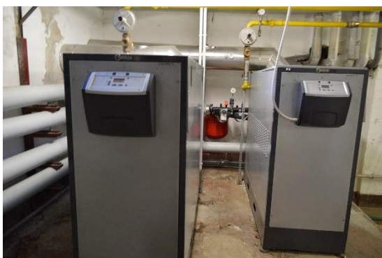
Figure 87 the methane condensing furnaces, part of the heating system.
