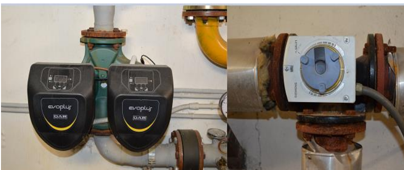
Figure 60 A-B: a twin pump and a three way valve
