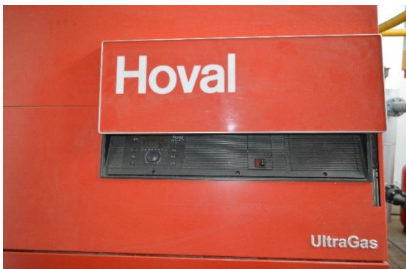
Figure 102 The condensing methane furnace of the thermal system I
