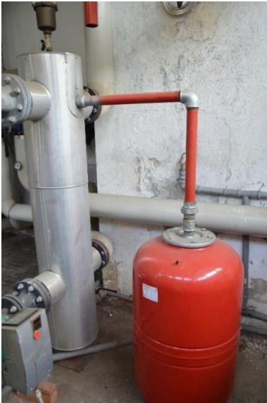
Figure 104 The expansion tank of the thermal system
