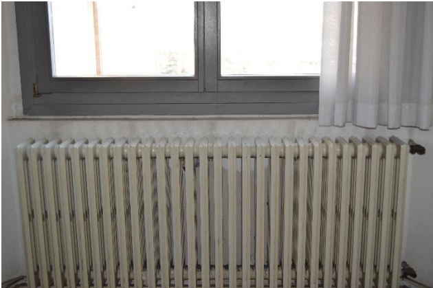
Figure 57 heating diffusion is provided by 101 radiators.
