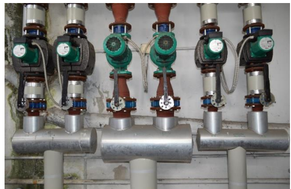
Figure 103 The electric pumps of the thermal system ☐
