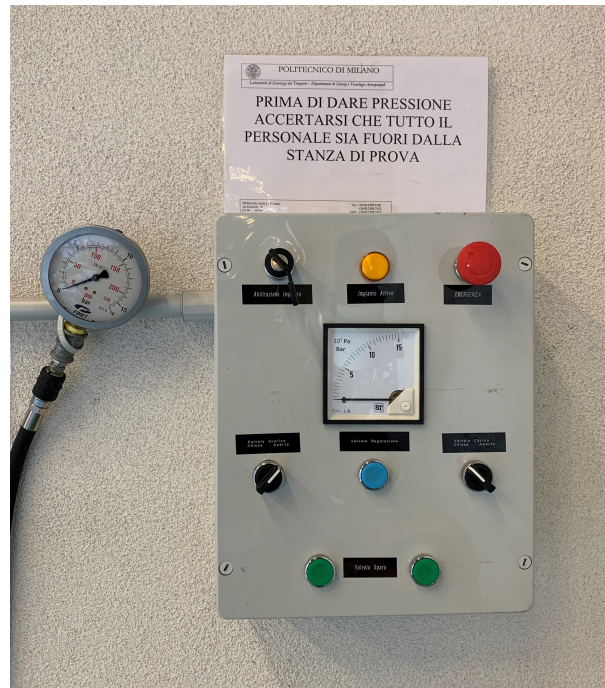
Figure 4.42: Exterior Control Panel
