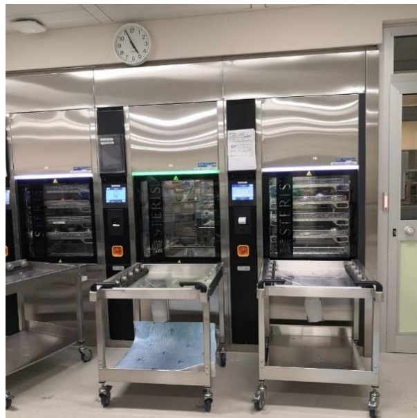
Fig. 18: end of the washing cycle (clean side of the CSSD)
