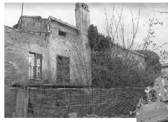
Abandoned Building E VIA MAZZINI
