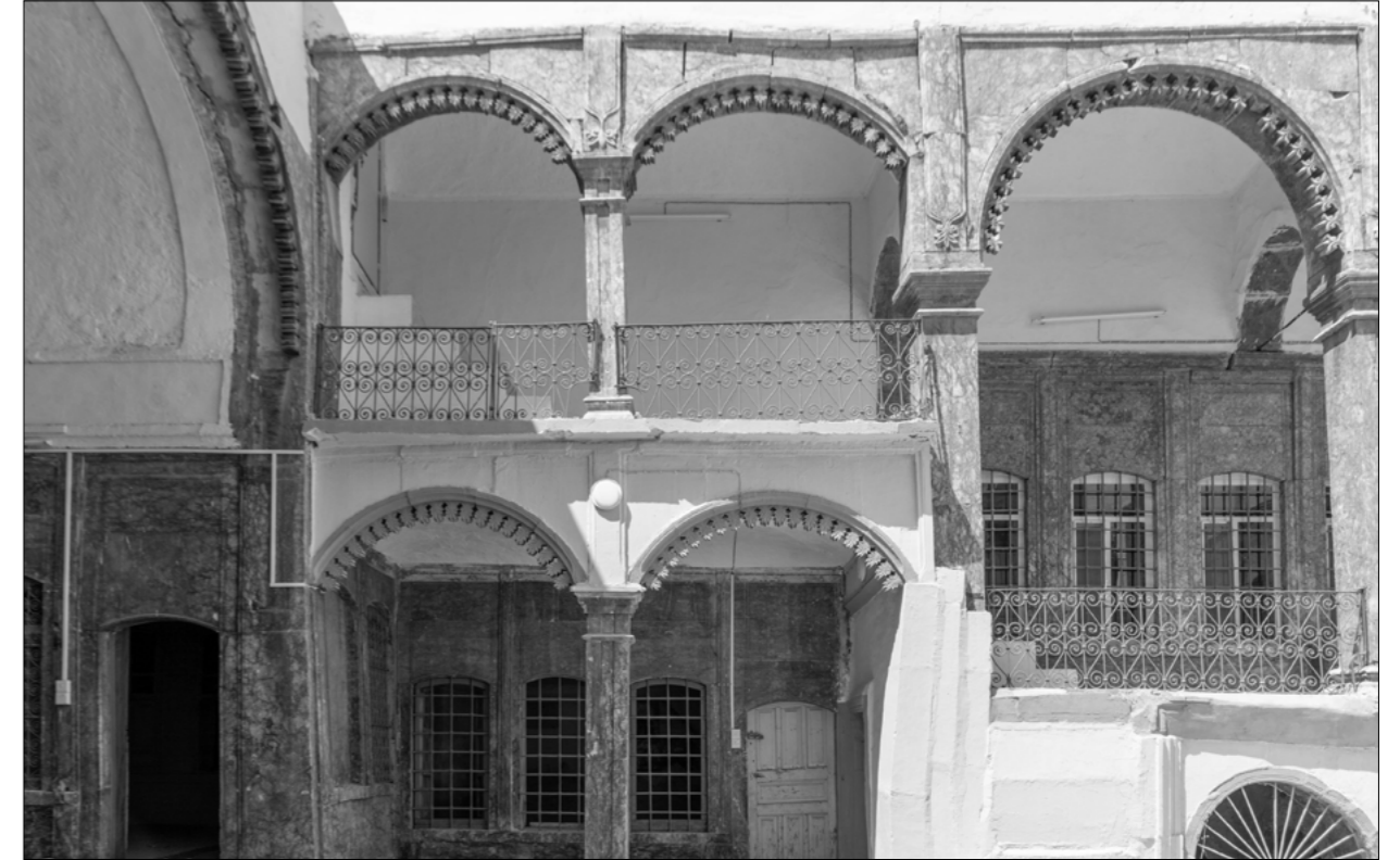
Fig.17 A rebuilt old Mosul house after its destruction showing the house court and the typical dicorative elements.image by Saad Haadi, June 2021.
