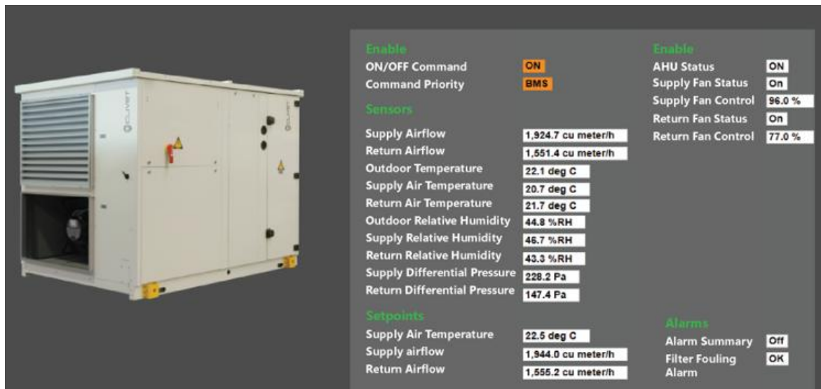
Figure 53: Example of AHU on the BMS interface – Source: case study documentation
