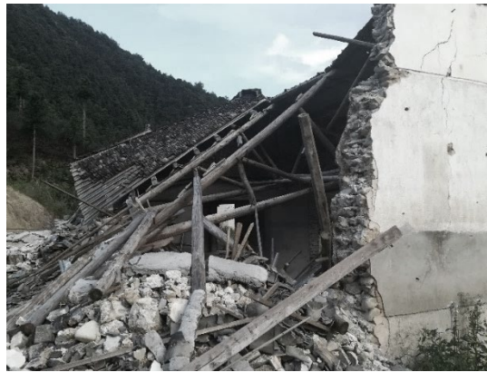
Figure 3-4 damage of structure (photo from author)
