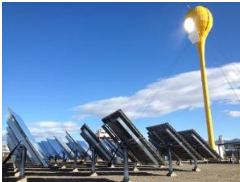
Figure 2-8: Aora Solar, Pilot CSP plant with a Solar-Hybrid micro-gas Turbine [29]
