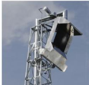
Figure 4-4: Jemalong Solar Thermal Station, Solar Receiver. [52]
