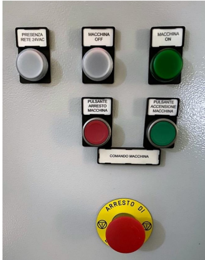
Figure 42: Control panel image
