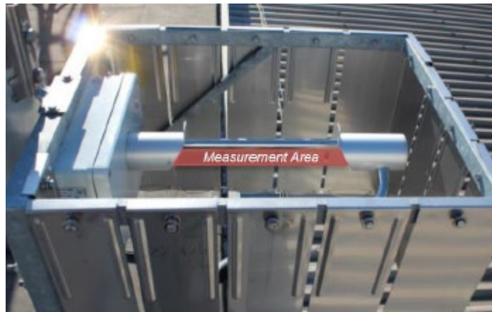
Figure 2-4 Disdrometer installed on the rooftop of Building 20 – Politecnico di Milano campus
