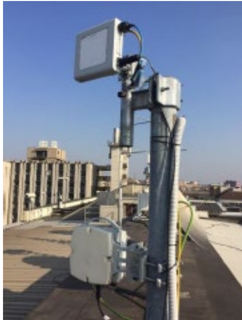
Figure 2-2 Huawei E-band and D-band transceivers installed on the rooftop of Building 20 of Politecnico di Milano.
