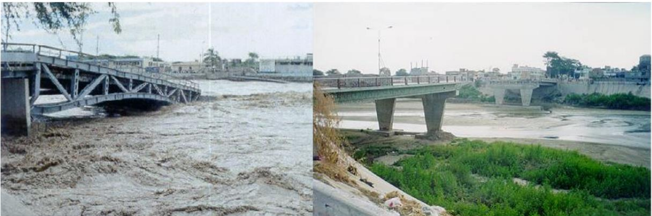
Figure 2. Collapsed bridges during the 1998 El Niño flood event at Piura River, Peru [30]
