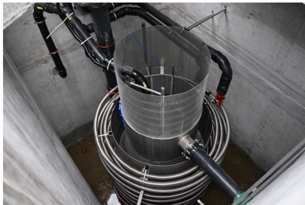
Figure 1.7: Example of an in sewer integrated heat exchanger installed directly within an urban sewer conduit [14].
