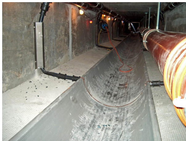
Figure 1.12: Example of an existing urban sewer conduit equipped with an integrated heat exchanger for wastewater heat recovery, as considered for the case study [15].
