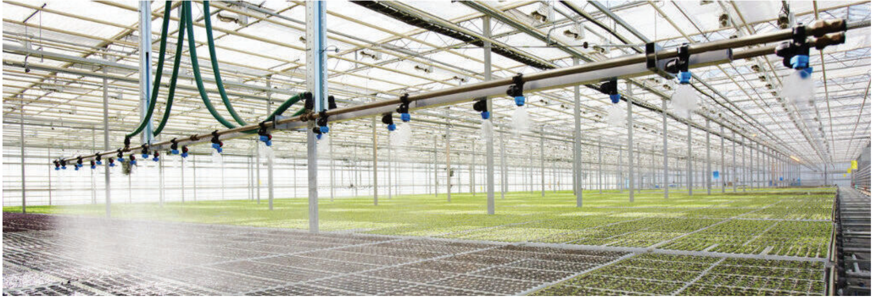
Smart watering system
