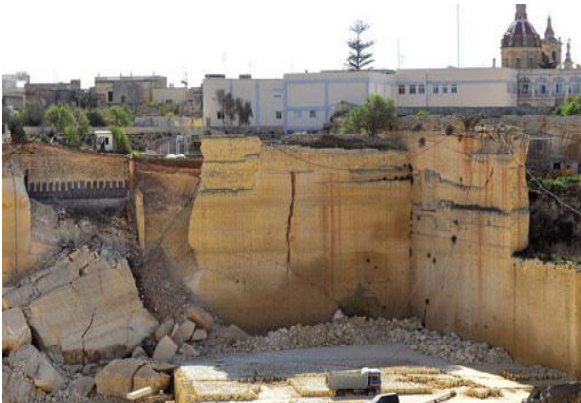
IMAGE_52 _Quarry Collapse Inside An Urban Area In Malta
