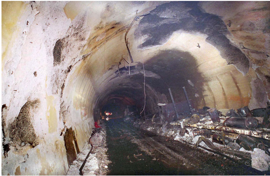
Figure 1: Effects of fire in Mont Blanc Tunnel, on March 1999. [Wallis, 2001]
