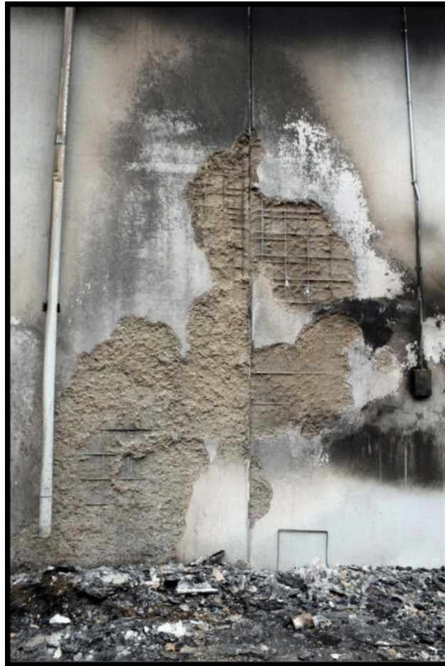
Figure 1.13: Fire spalling on an external concrete wall [McNamee, 2013]
