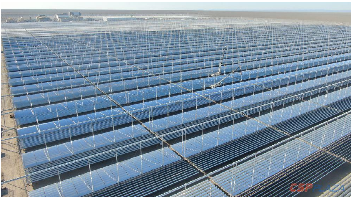
Figure 1-9 Lanzhou Dacheng Dunhuang plant in China.
