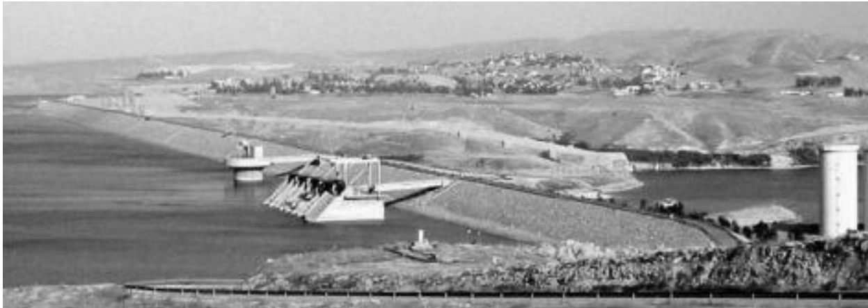
Fig. 2.10 The Mosul dam, 2011, Completed in 1984, the dam suffers from structural problems that caused the U.S. Army Corps of Engineers to once call it 'the most dangerous dam in the world,' an accusation rejected by Iraqi authorities.
