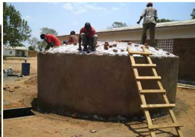
Figure 6-6 Above ground tank
