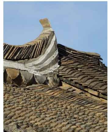
Fig. 5.30 Ridge decoration of the roof, in this case both the tiles and the stone decoration are present
