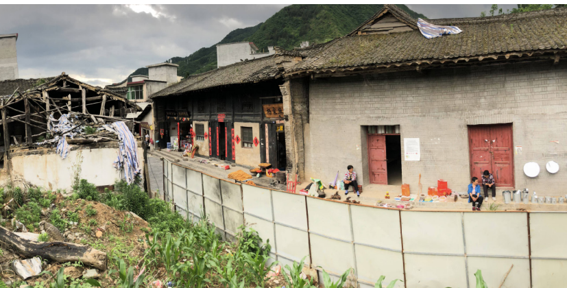
Fig. 6.8 Panoramic view of the “lacuna”, is possible to see the traditional structural system in the remainings of the courtyard.
