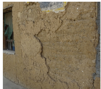
Fig. 5.25 A wall with earth-based plaster, subject to plaster peeling phenomena
