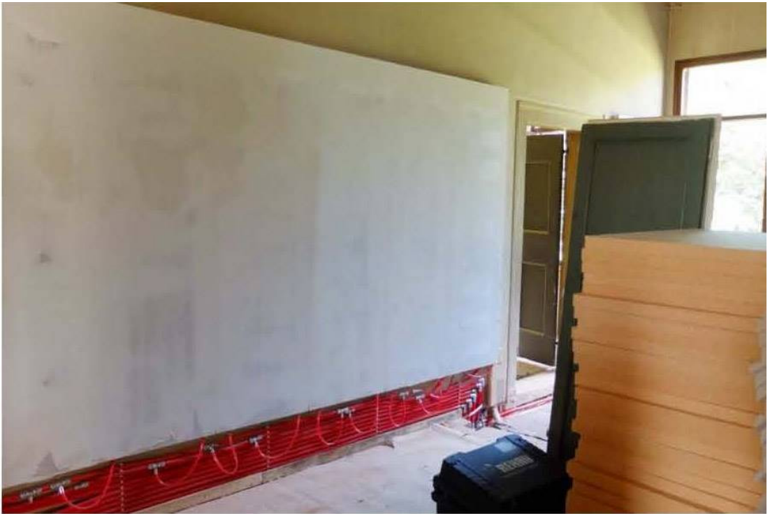
Fig. 3.17 Photo of the wall mounted radiant system
