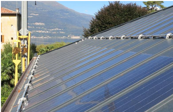
Fig. 3.23 (on the left) Photovoltaic system of the roof of the Villa
