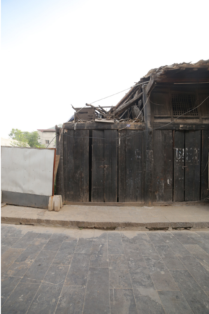
Fig. 6.7 Photograph from the ancient road, is possible to notice the collapsed part of the courtyard.
