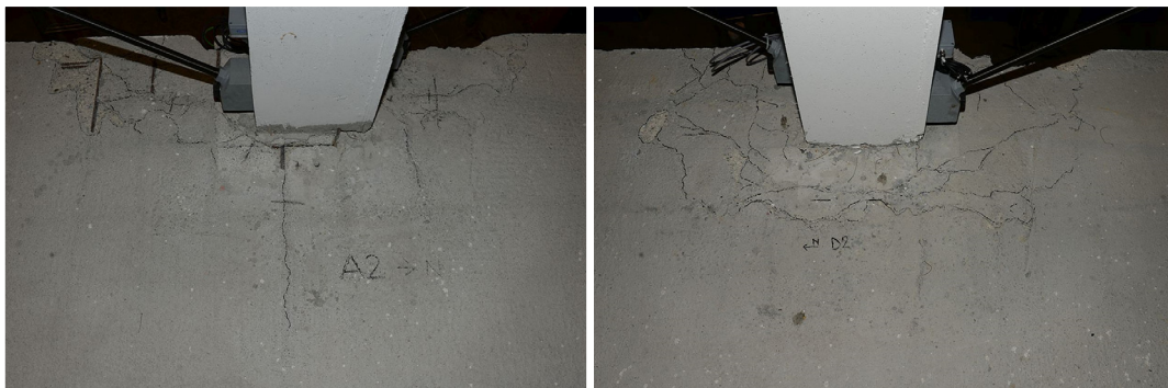
Figure 7.44 Damage in the slab-column connections, 1 st floor a) A2, b) D2.
