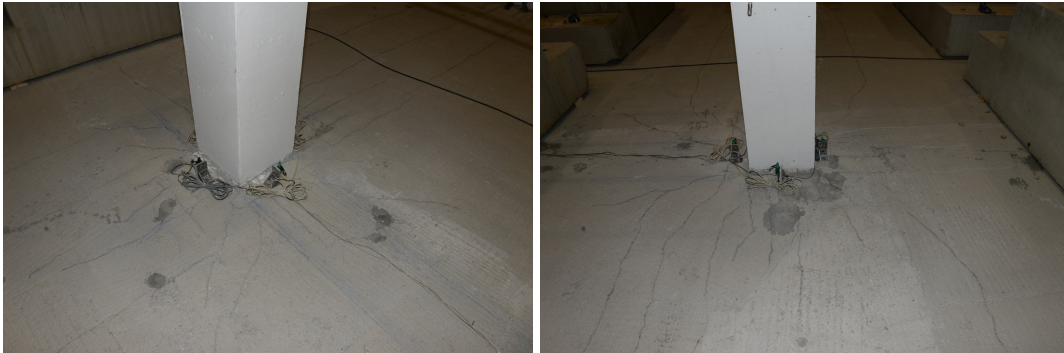
Figure 8.34 Radial cracking in the internal connections on the 2 nd floor a) B2, b) C2.
