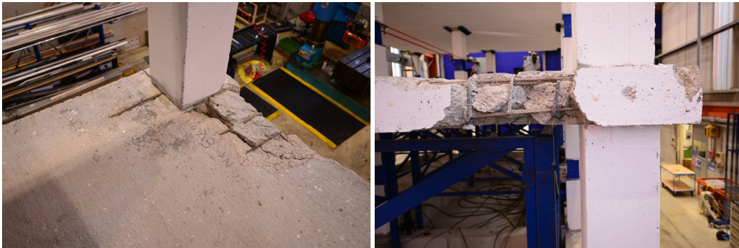
Figure 8.24 A3 connection after test Cyc-2 (g04), a) slab-column connection, b) slab west side.
