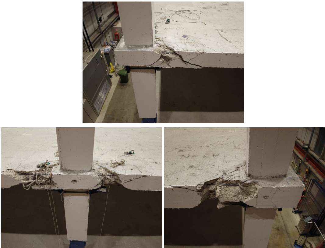
Figure 8.31 Damage in the A alignment in the 2nd floor, a) A1, b) A2, c) A3.
