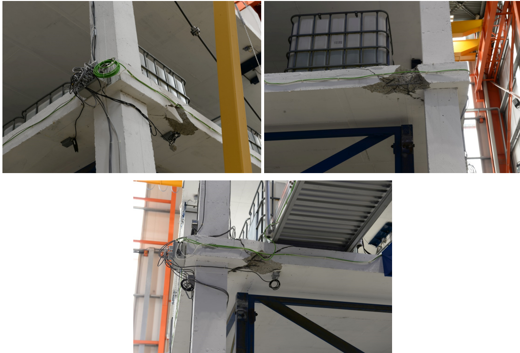
Figure 7.38 a) A1, b) D1 and c) D3 connections after the 2.5% drift, tests B1 (f02).
