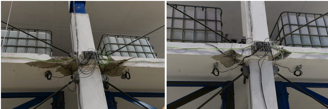
Figure 7.39 a) A2 and b) D2 connections after the 2.5% drift, tests B1 (f02).
