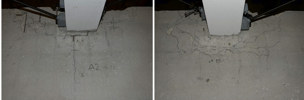
Figure 7.40 a) A2 and b) D2 slab-column connections after the 2.5% drift, tests B1 (f02).
