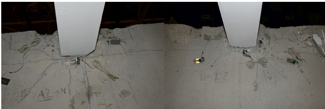
Figure 8.33 Cracking in 2 nd floor, connections a) A2 west side and, b) D2 east side.
