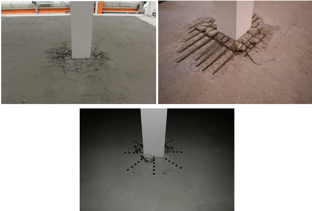
Figure 8.45 B2 a) before and b) after the removal of the damaged concrete pieces and c) C2 connections at the end of the test CYC-2 (g04).
