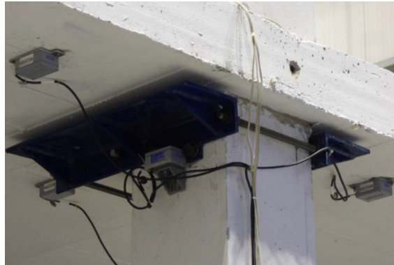
Figure 4.54 Inclinometer positioning and safety system.
