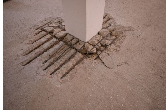
Figure 9.37 SlabSTRESS B2 connection east-west direction after the removal of damaged concrete pieces.
