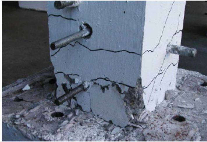
Figure 9.17 Kang and Wallace, 2004 [5] damage at the column base of the RC specimen.
