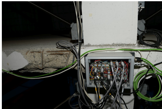
Figure 4.16 Data acquisition box.
