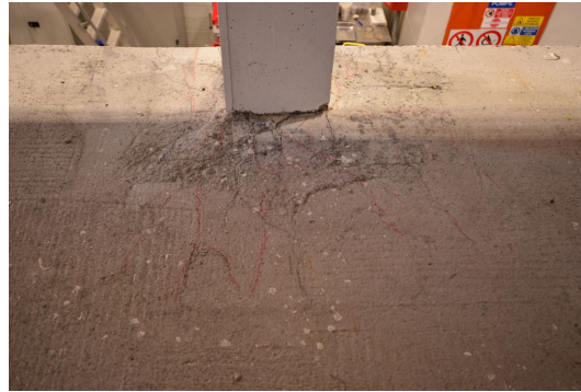
Figure 9.33 SlabSTRESS 1 st floor slab damage, edge parallel to lateral load direction, connection a) B1 north, b) B3 and c) C3.
