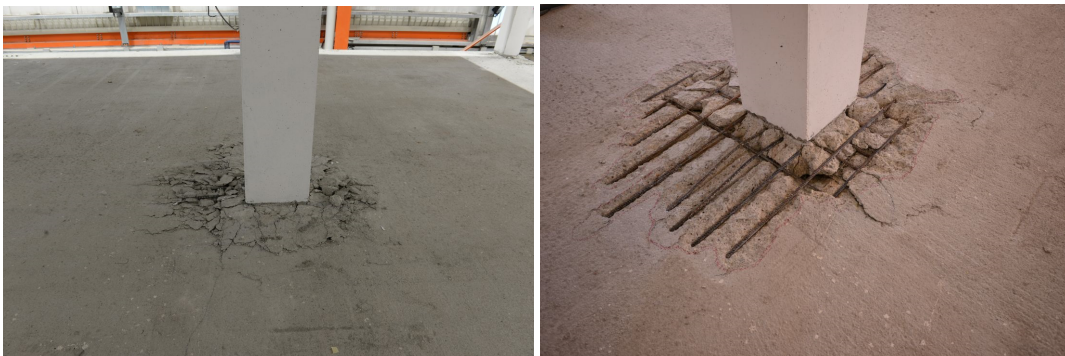
Figure 8.28 B2 connection after test Cyc-2 (g04) a) north-south direction before the removal of the damaged concrete pieces and b) east-west direction after the removal of the damaged concrete pieces.
