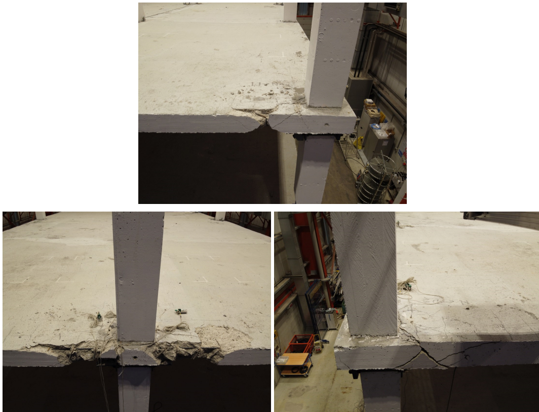
Figure 8.32 Damage in the D alignment in the 2nd floor, a) D1, b) D2, c) D3.
